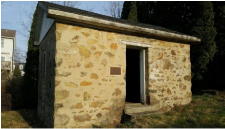
This View Shows Severe Deterioration
